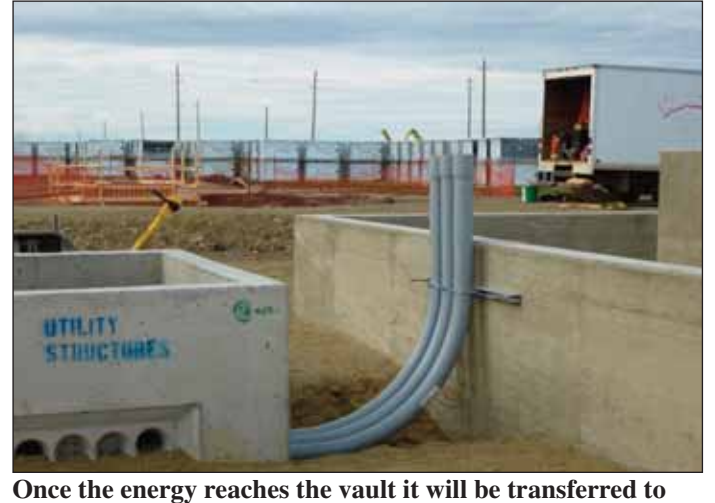
Once the energy reaches the vault it will be transferred to the ON Hydro lines and sent to the distribution centre in Barwick.
