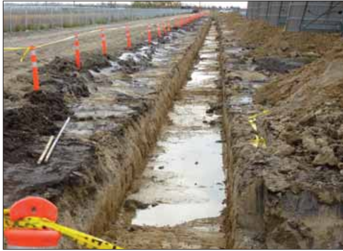
Trenches are dug between the pilings. The panels connect to wires which travel along a trough to collector panels situated between the rows of panels. These then connect to cables that are laid into the troughs ending at the vault.
