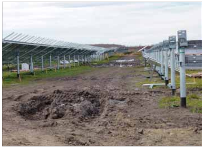
Pilings, or screws, waiting panels, beside a road before gravel was used. It was easy to understand, after seeing this, why there have been gravel trucks going into the sites all summer.
